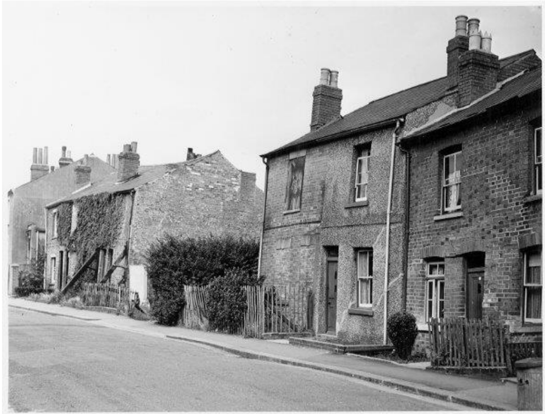
Mining subsidence at Field Road, Reading, September 1951. Photograph from Reading Chronicle Collection (REDMG 1980.36.B395.2c).
